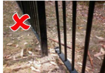
A fence in disrepair can lower the effective height of the barrier or provide a gap for a child to enter the pool area.
