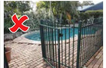
Do not tie or prop open a gate when it's not being used.
