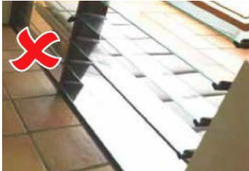
Louvres with a gap of more than 100 millimetres do not comply.
