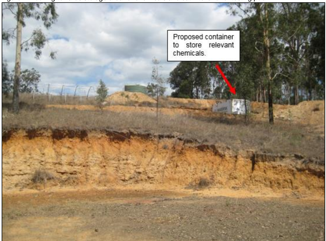
Figure 7: Looking towards storage area for chemicals and cut into land for testing pad
