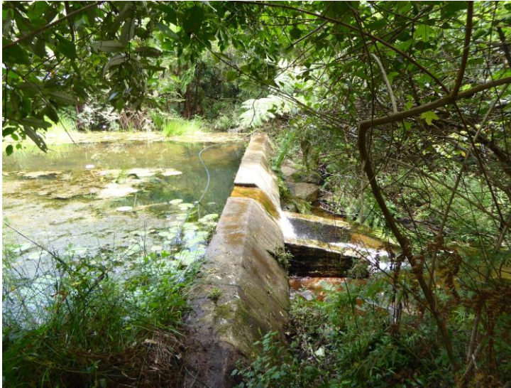
View over the concrete weir from the eastern bank of Plunkett Creek.
