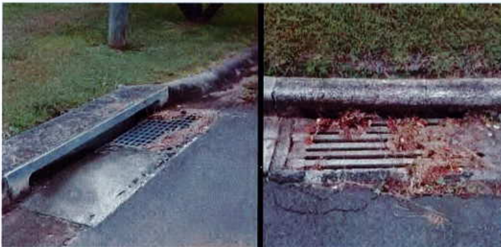
Figure 2-1 Blocked Stormwater Inlets at Kalbar
