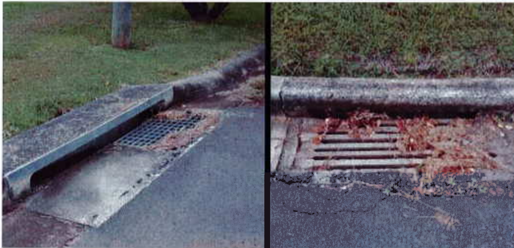
Figure 2-2 Example of Blocked Stormwater Inlets
